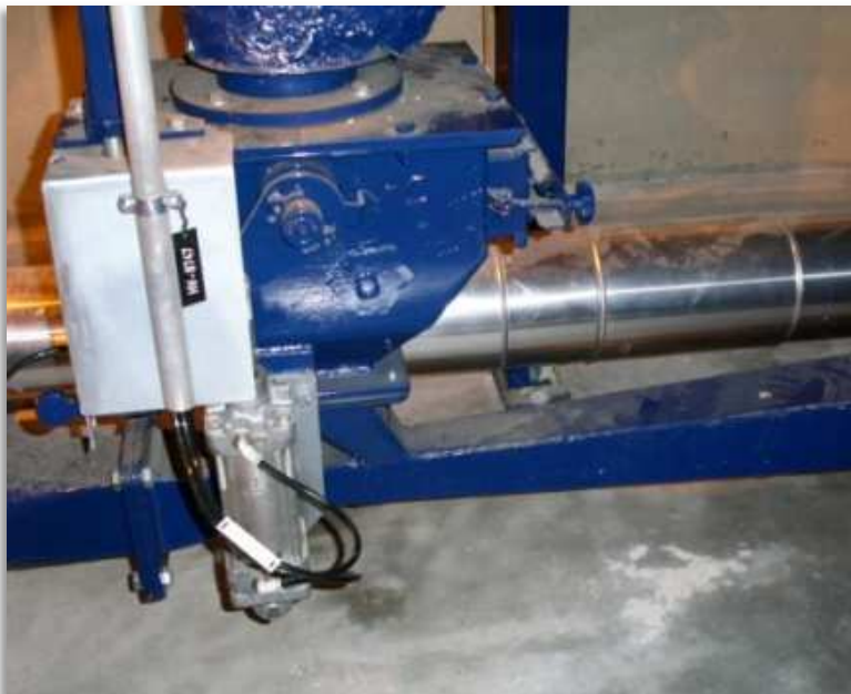
Feed valve and injector
